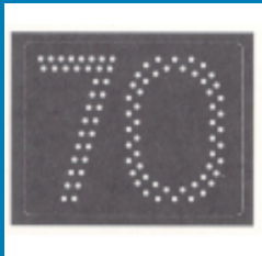
Speed limit displayed on a display panel
